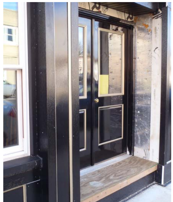
Parcel #13: Exposed insulation; exposed wood.
