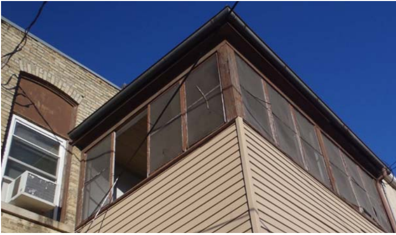
Parcel #30: Peeling paint; rear porch in poor condition.
