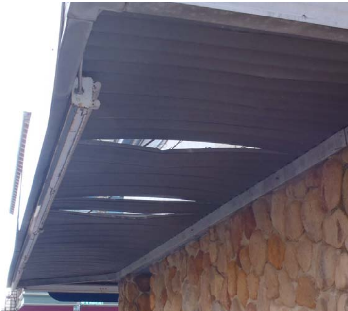
Parcel #17: Metal awning in poor condition.
