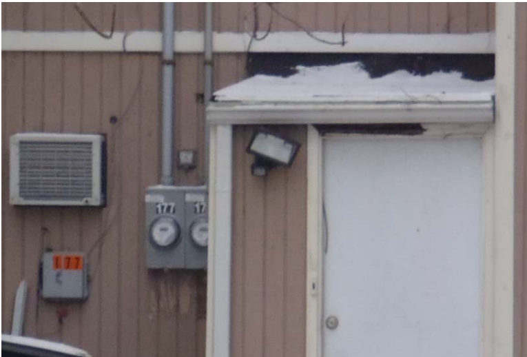
Parcel #32: Exposed wood; doorframe in poor condition.
