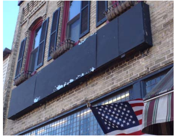
Parcel #31: Boarded up, peeling sign cabinet.
