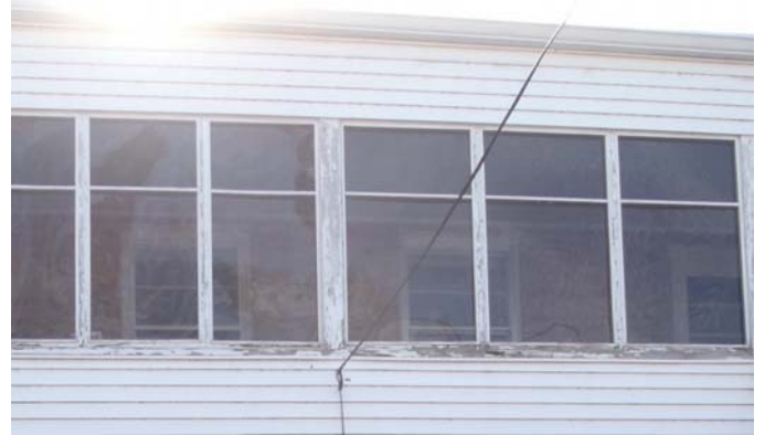
Parcel #54: Exposed wood, peeling paint.
