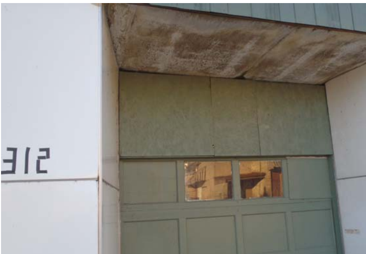
Parcel #19: Taped on address, fiberboard façade, peeling paint, exposed wood.
