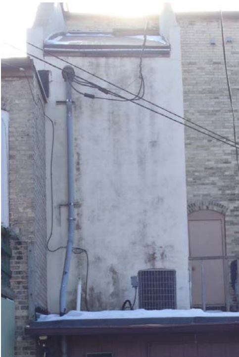
Parcel #55: Dirty/mildew stucco façade.
