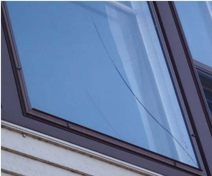
Parcel #9: Cracked window.
