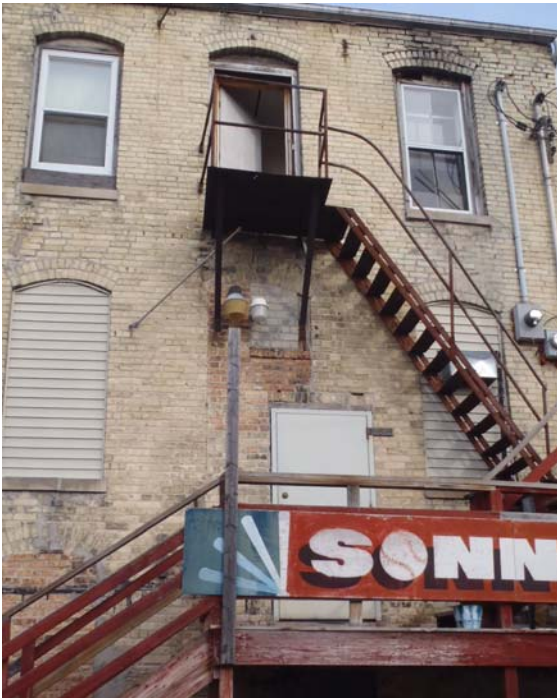
Parcel #66: Bricked/boarded up windows; peeling paint, exposed wood; tuckpoint needed.
