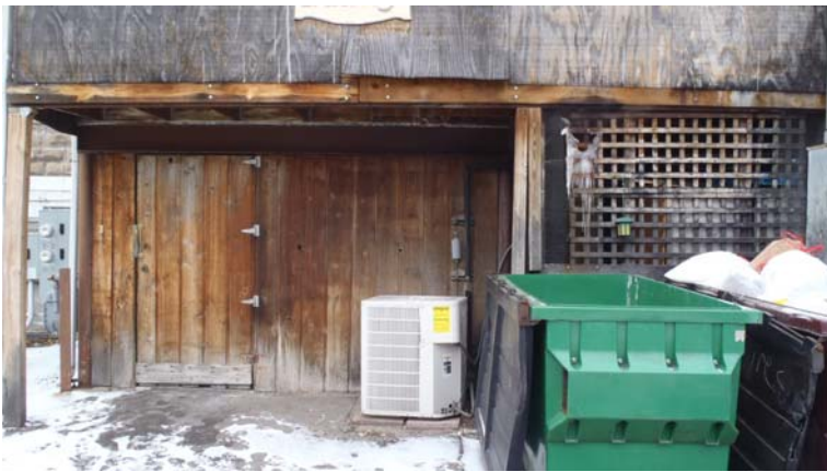
Parcel #93: Exposed wood; peeling plywood.
