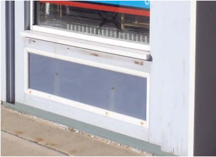
Parcel #15: Rusting nails on façade.
