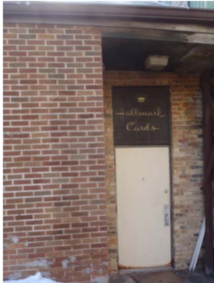
Parcel #51: Exposed wood trim; rusted door bottom.
