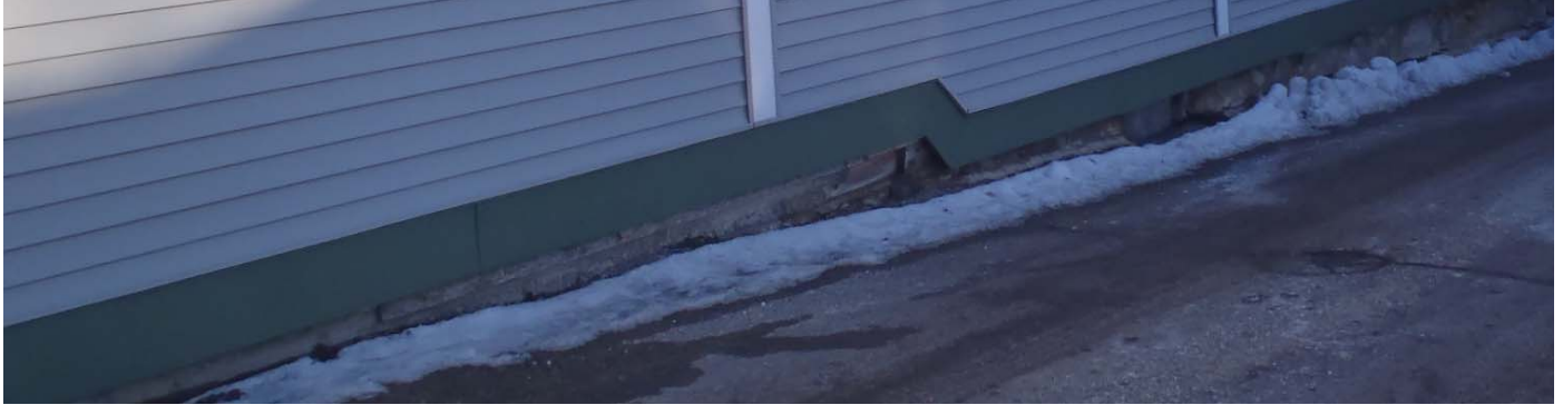
Parcel #8: Foundation in poor condition.
