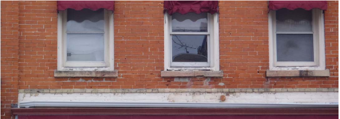
Parcel #65: Window frames and bricks below windows in poor condition.
