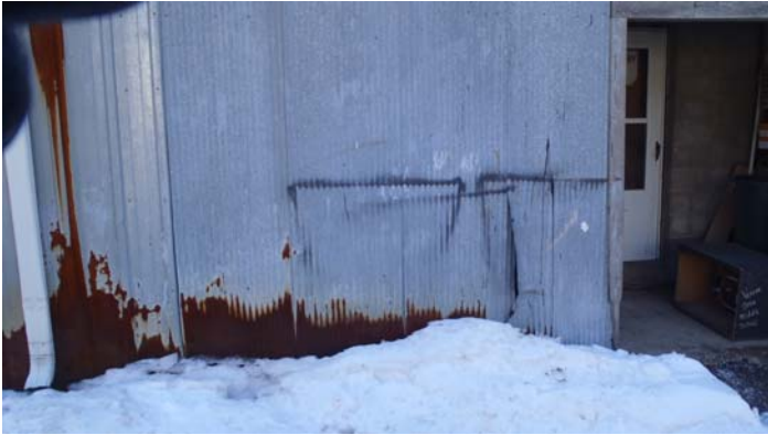
Parcel #53: Rusted corrugated metal façade.
