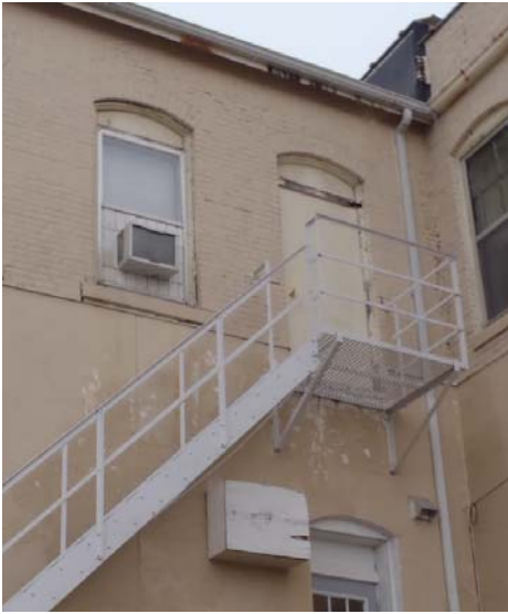
Parcel #90: Peeling paint, boarded up vent, rusty gutters.
