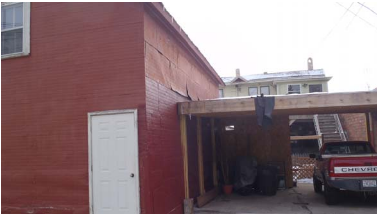
Parcel #103: Peeling sheet metal siding; exposed wood/ fiberboard carport (top).
