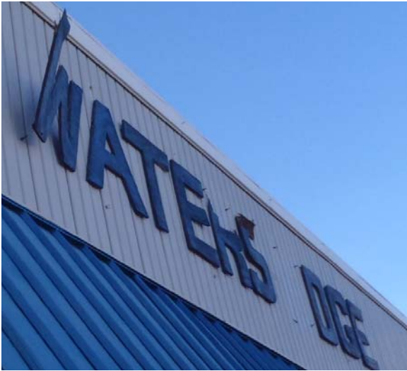
Parcel #21: Dilapidated plywood sign.
