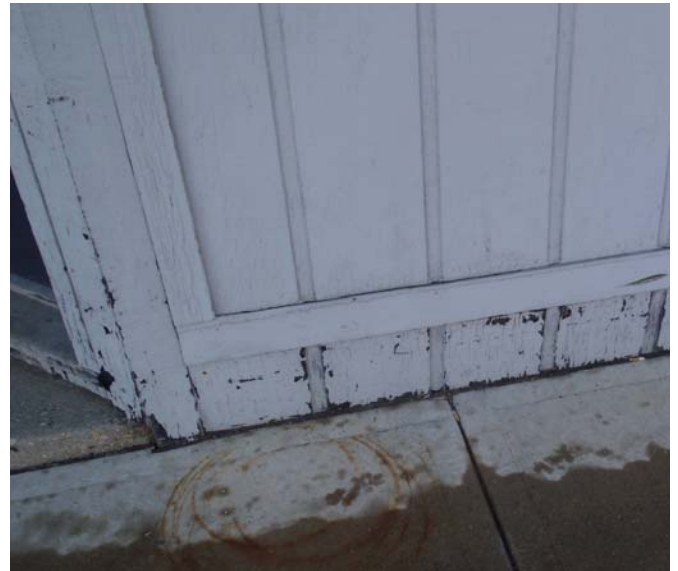
Parcel #10: Peeling paint.
