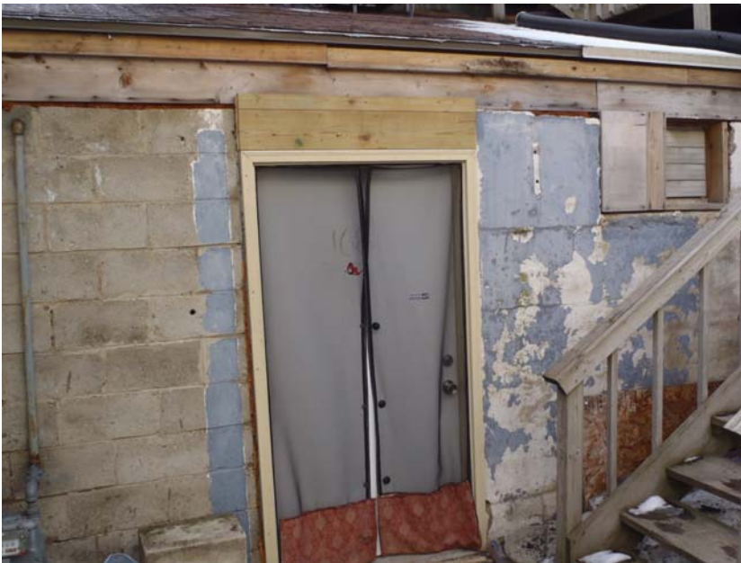
Parcel #27: Exposed wood, peeling paint.
