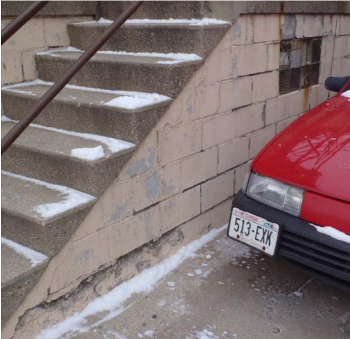
Parcel #60: Peeling paint, crumbling cinderblock, broken glass bricks.
