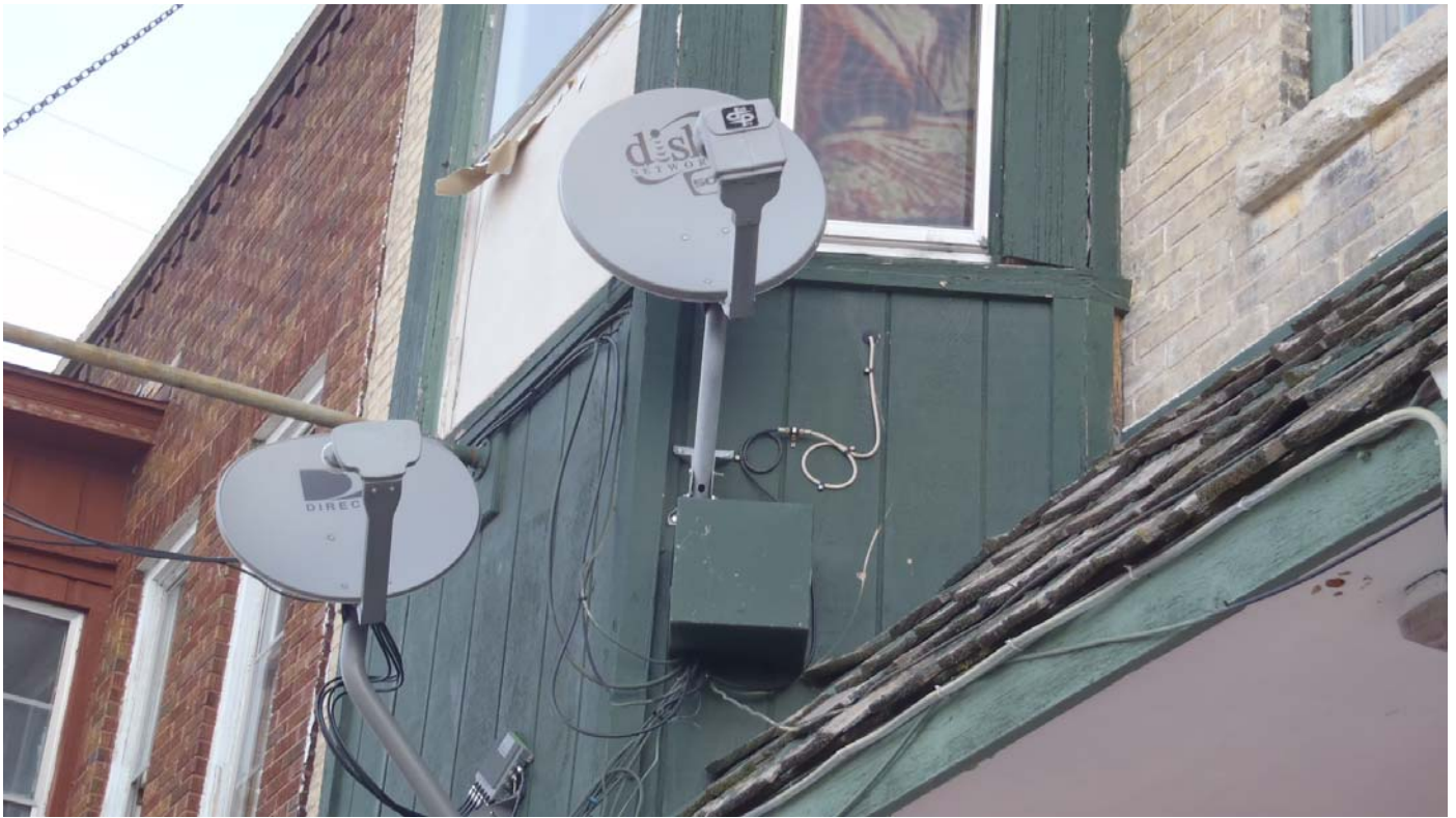
Parcel #73: Exterior wiring; shingles in poor condition; blocked window; loose wood siding.
