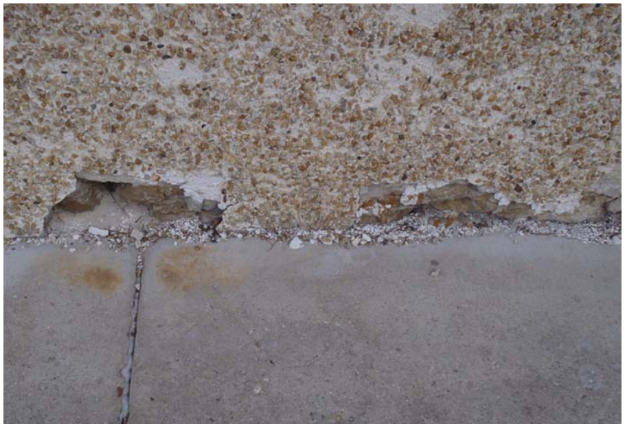
Parcel #48: Crumbling façade at base of building.
