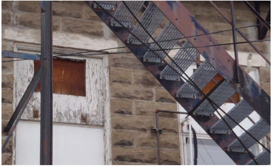
Parcel #92: Exposed wood; boarded up windows.
