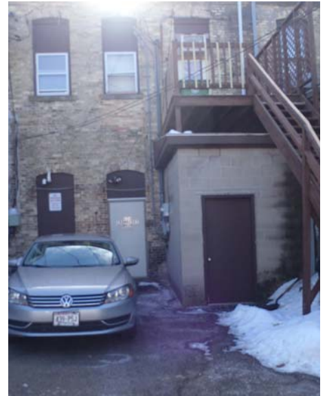
Parcel #52: Exposed cinderblock façade; partially boarded windows.
