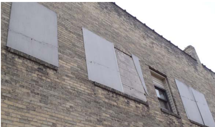
Parcel #88: Boarded up windows.
