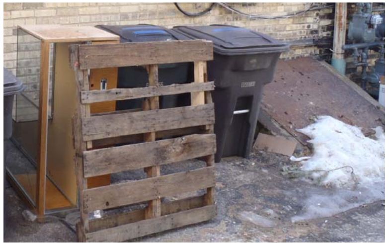
Parcel #25: Pallets & junk in rear; rusty basement door.
