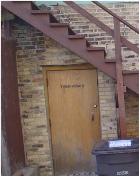
Parcel #50: Rear door in poor condition; façade cracks; tuckpointing needed.
