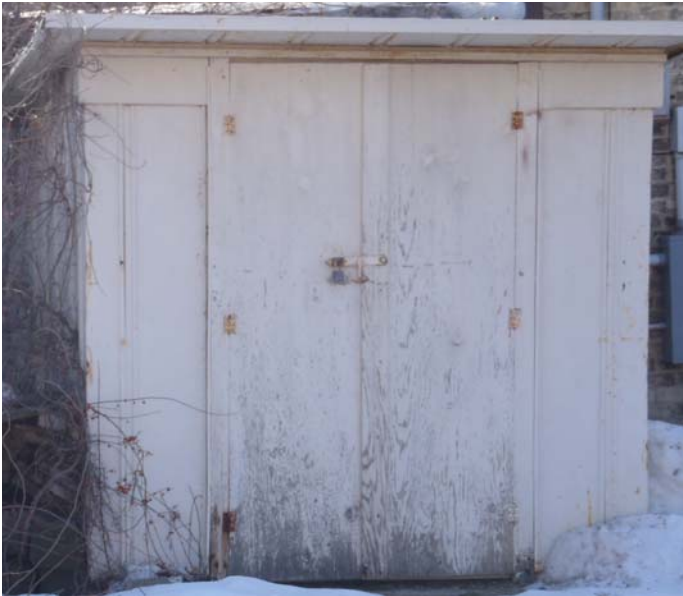
Parcel #57: Peeling paint, exposed wood, rusted hardware on shed.
