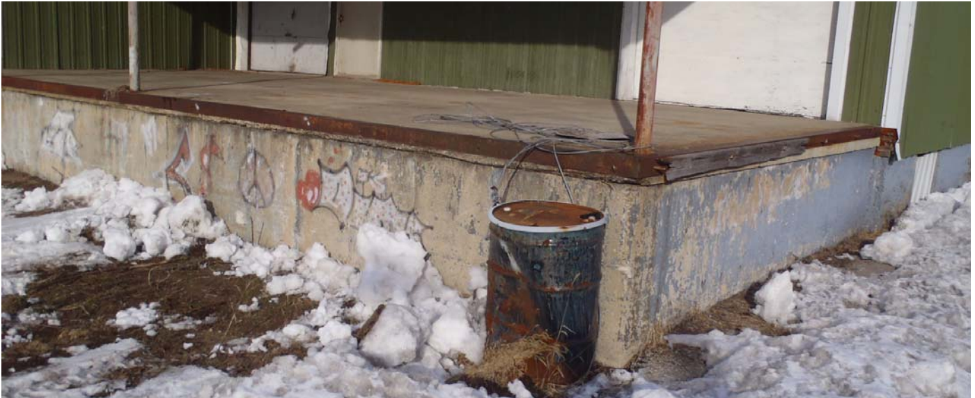
Parcel #41: Rusted barrel, graffiti.
