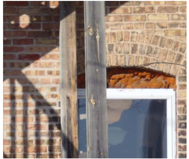
Parcel #33: Exposed foam at top of windows.
