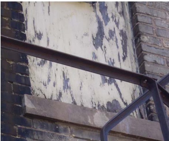
Parcel #24: Boarded up rear window.
