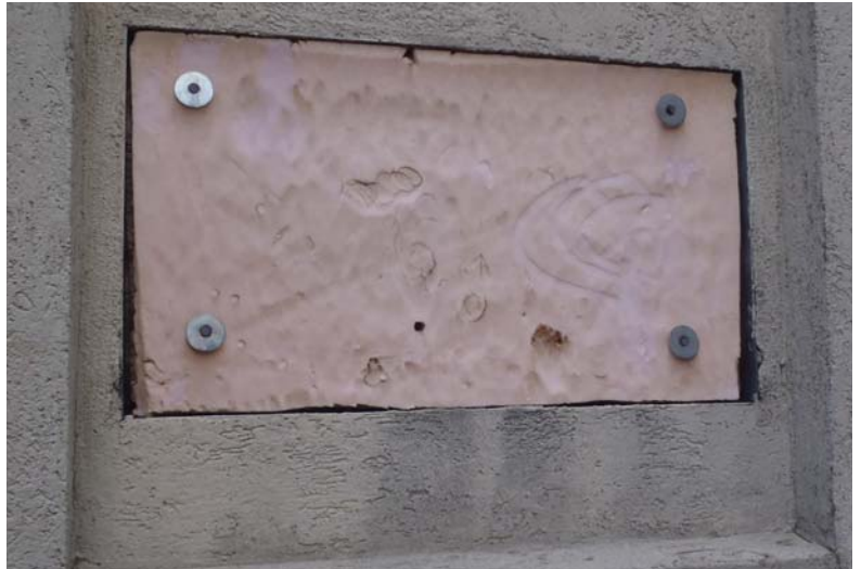
Parcel #23: Holes in EIFS façade.
