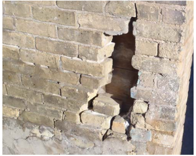
Parcel #16: Crumbling façade.
