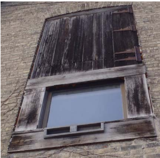
Parcel #71: Peeling paint; exposed wood.
