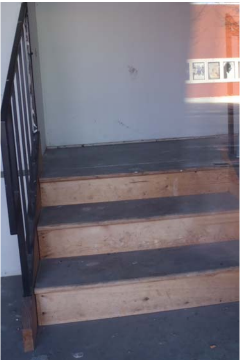
Parcel #37: Interior ground floor in poor condition.
