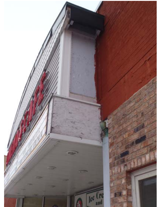
Parcel #29: Peeling paint; fiberboard façade.
