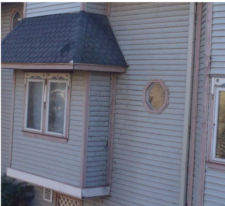
Parcels #11-12: Façade mildew/dirt.
