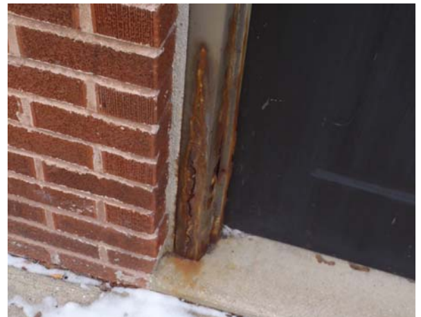
Parcel #89: Rusted doorframe.
