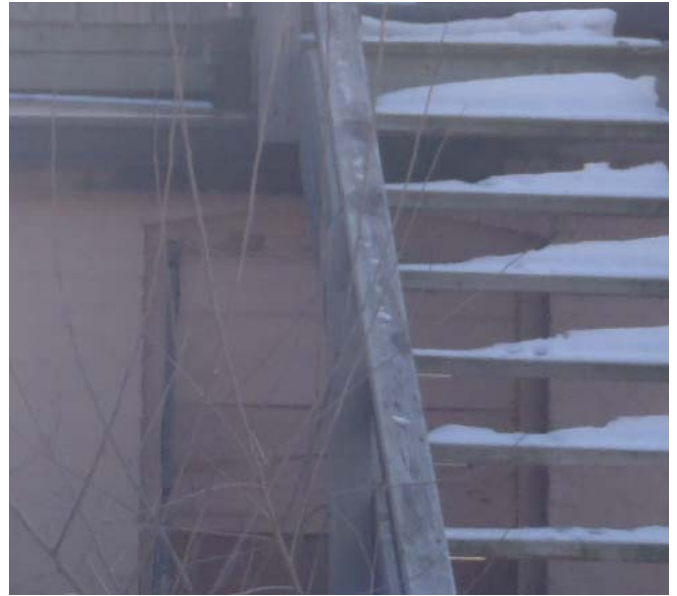
Parcel #58: Partially boarded up window.
