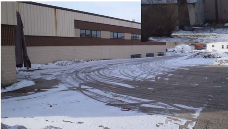
Parcels #79-82: Rusted façade; little/no buffer between driveway and street along portions of parcels (left).
