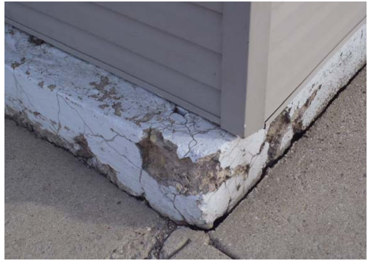
Parcel #75: Crumbling foundation.
