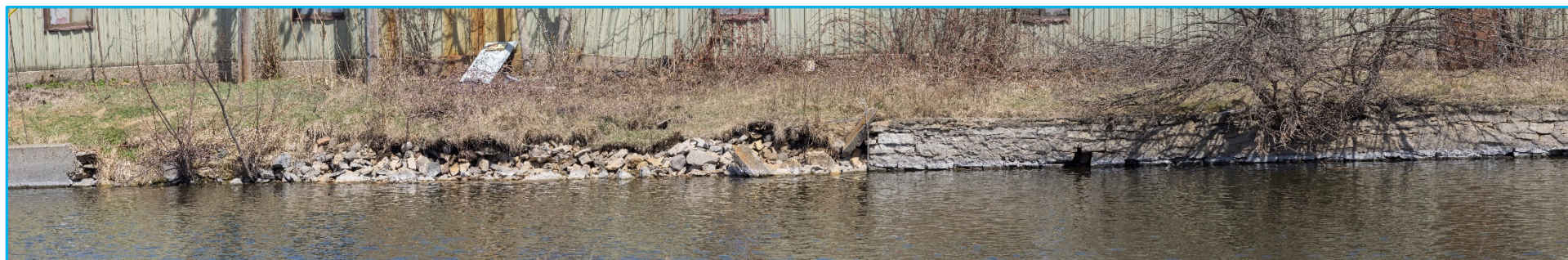
FIGURE 9: THE YAHARA RIVERBANK HAS DETERIORATED AND BECOME UNSTABLE.
