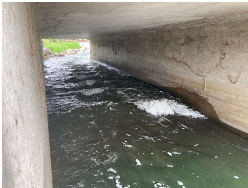
Figure 5. Existing box culverts under 4 th St. Date: May 18, 2022. Approximate discharge at Forton St gauge: 315 cfs, approximate single culvert flow 105 cfs.
